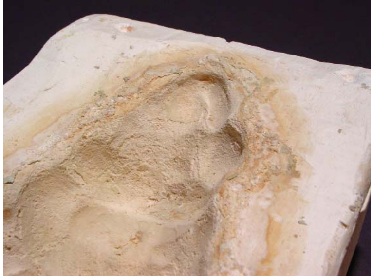
Detail of damage caused by salts
